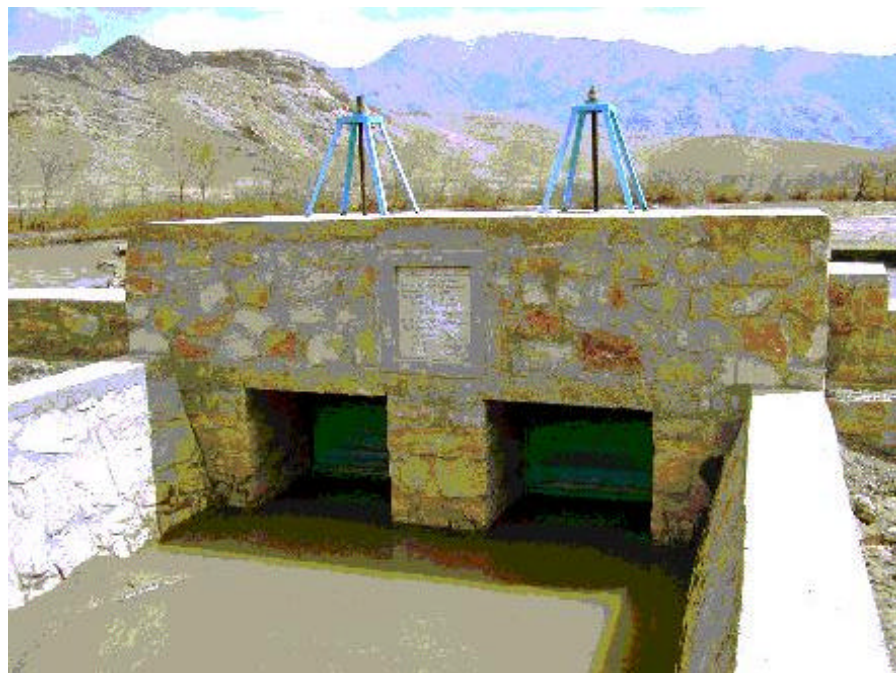
Figure 2.7. A typical gate-fitted canal intake
