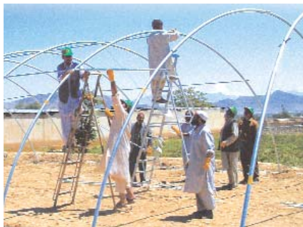
Installation of greenhouses at the Protected Agriculture Center (PAC), Badam Bagh Research Station, in Kabul, Afghanistan.
